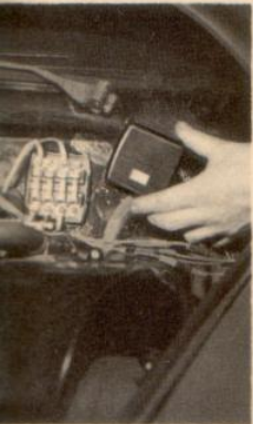
Fuse box (left side)
